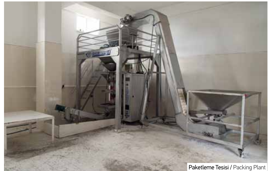
Paketleme Tesisi / Packing Plant
